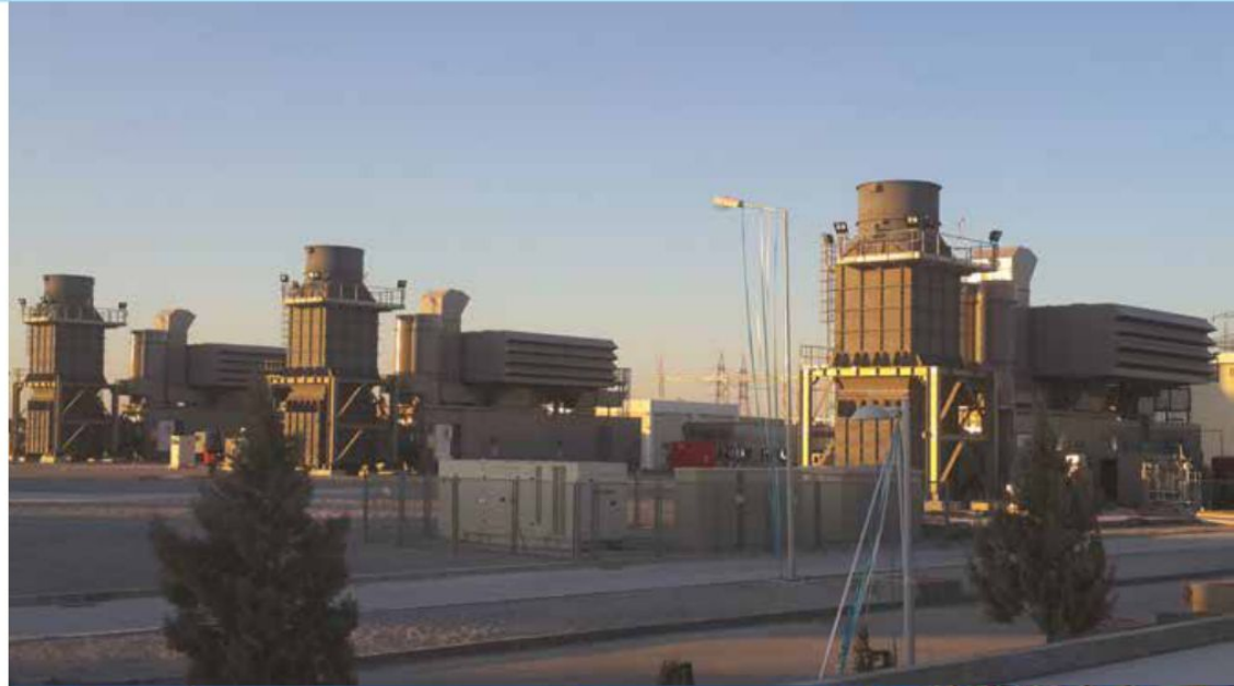
AHAL POWER PLANT / TURKMENISTAN
